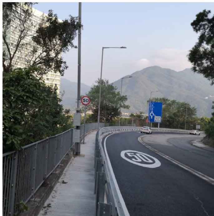
Installation of roadside safety barriers with slender size on Tai Po Road — Ma Liu Shui
