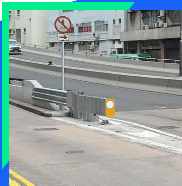
Installation of crashworthy end terminal at a diverging point on Wong Chuk Hang Road
